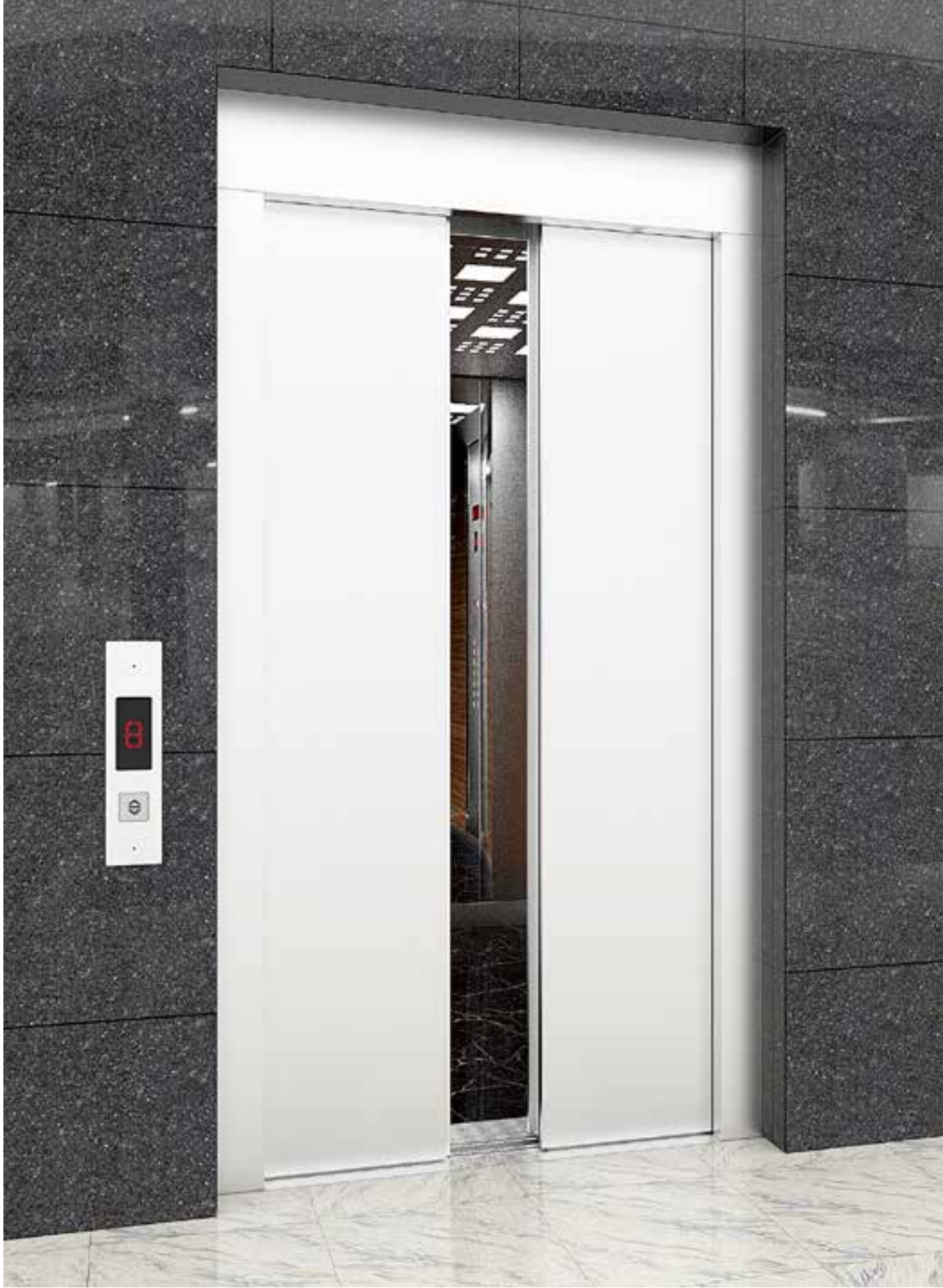
2 Panel Merkezi Kapi 2 Panel Central Elevator Door
